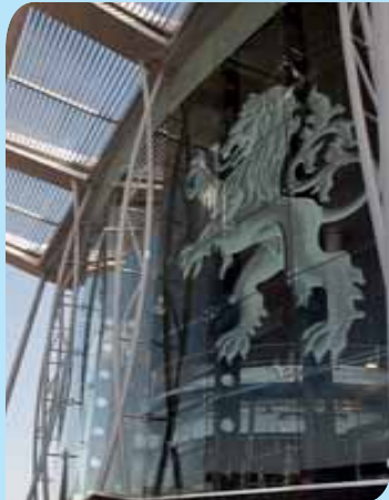
Lion Nathan's new facility in South Auckland is taking shape. It will have an annual capacity to produce 180 million litres of beer.
