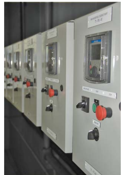
A neat row of new Variable Speed Drive control cabinets installed and wired to dosing pumps
