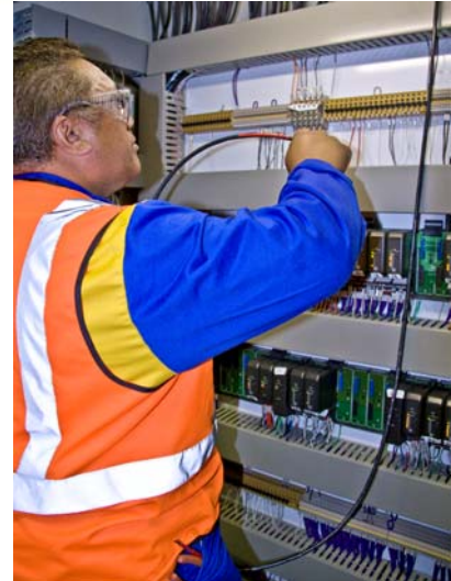
Electrix Technician prepares to wire in a new circuit to the PLC control cabinet
